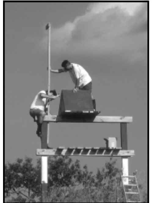
Shawn Padgett (standing) and Richard Bartlett work on a Peregrine tower. Repair and management of nest boxes and towers requires a tremendous number of man hours each year. Photo by Bryan Watts.
